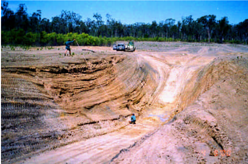
PHOTOGRAPH 5-3 – DEEP CUT-OFF TRENCH WITH SEEPAGE IN BED
