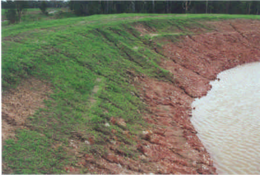
PHOTOGRAPH 5-7 - POORLY DISTRIBUTED TOPSOIL COVER
