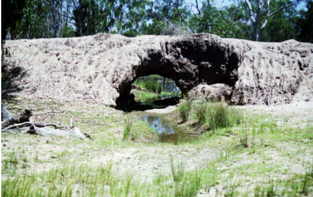
PHOTOGRAPH E-2 – DAM FAILURE DUE TO DISPERSION
