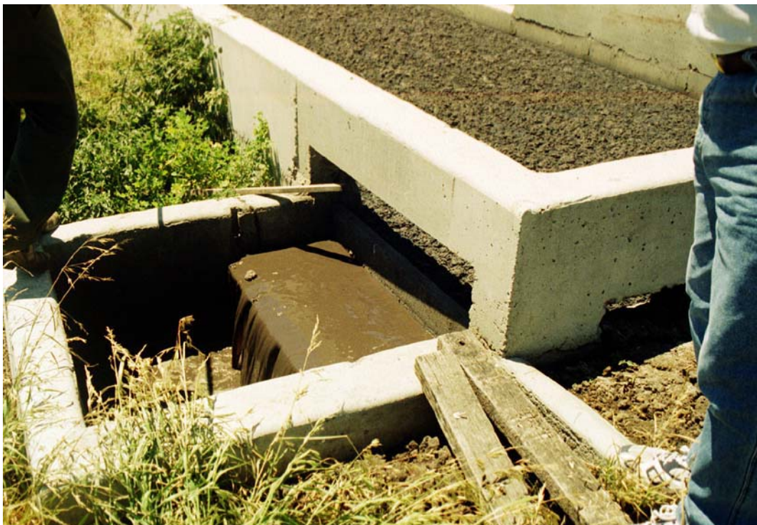
PHOTOGRAPH 1-4 - OVERFLOW WEIR WITH SCUM BOARD
